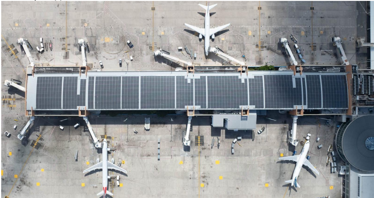
Solar Project at SIA: Aerial view of the Solar Photovoltaic (PV) system installed on the roof
